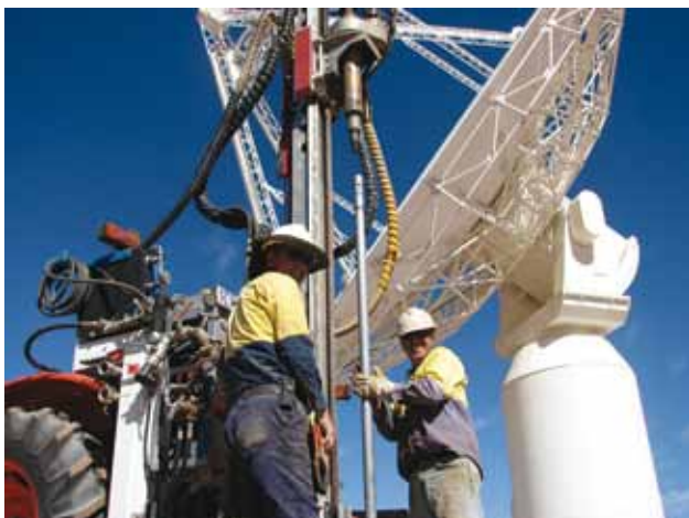
The Dongara Drilling team at the site of ASKAP Antenna 1 during the installation of the trial geo-exchange system. Image Credit: Graham Allen, CSIRO.
