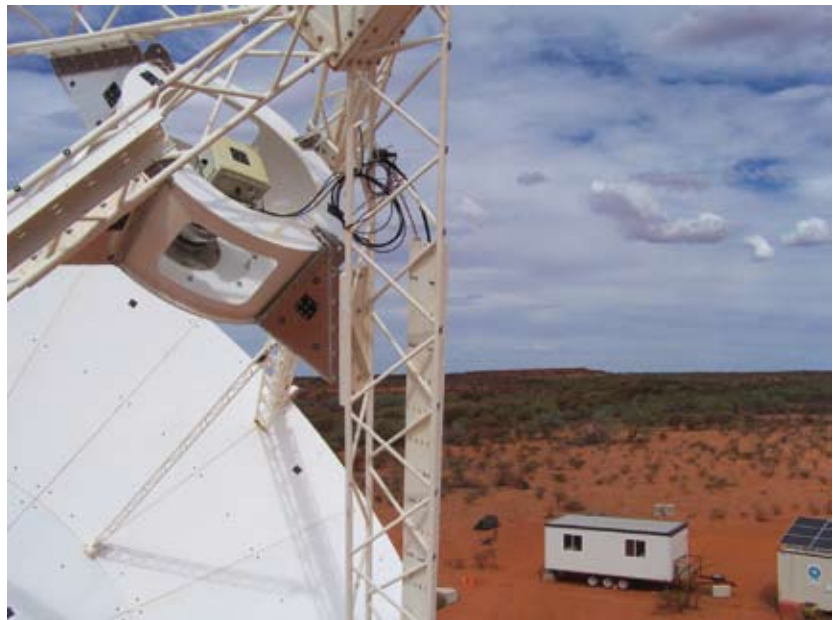
The completed feed installation. Credit: R Forsyth, CSIRO
