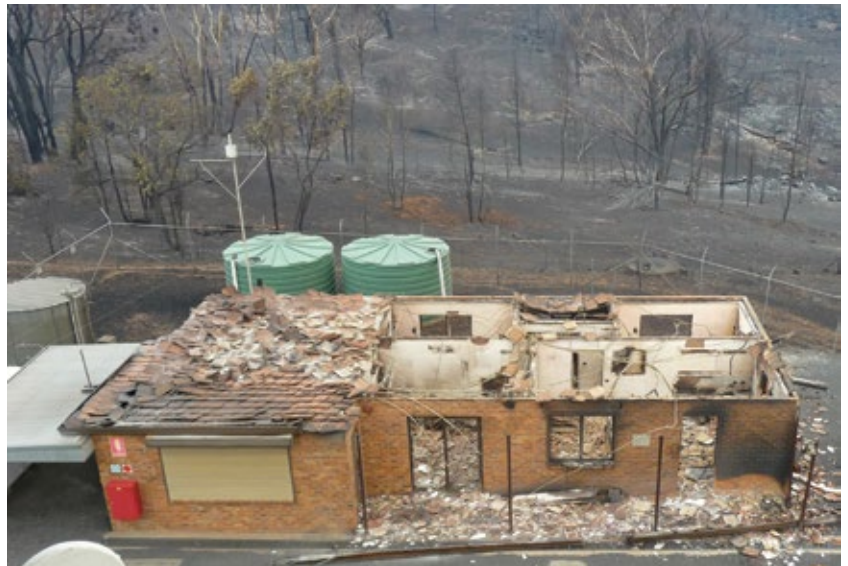
The main control room of the control building (at left), protected by its self-contained concrete structure and radio-frequency interference screening around the door and windows, is largely intact, however, the accommodation, office and living areas have been ruined.
