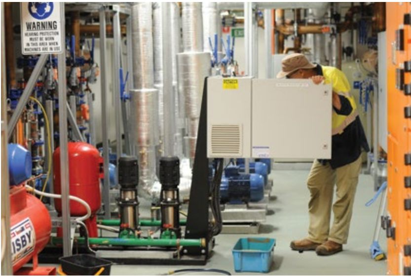
John Morris working in the plant room of the MRO Control Building following handover and occupation in late 2012.
