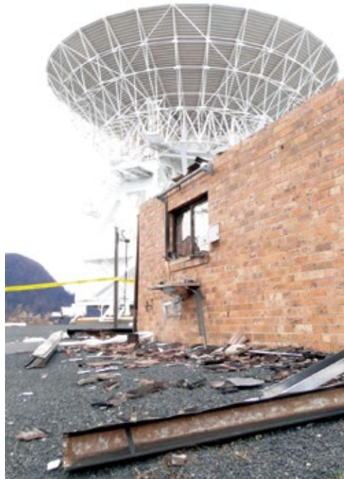
The Mopra antenna remains intact with very little evidence of damage but there has been significant damage to the control building.
