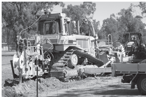
Figure 2: A cable-laying machine burying the broadband fibre near the central area of the Narrabri Observatory.
