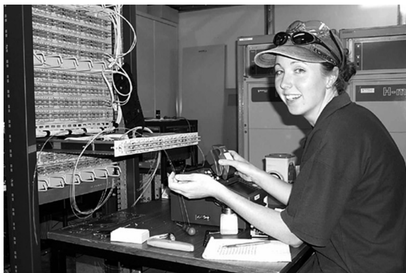
Leigh splicing fibres at the new patch panel in the screened room.
