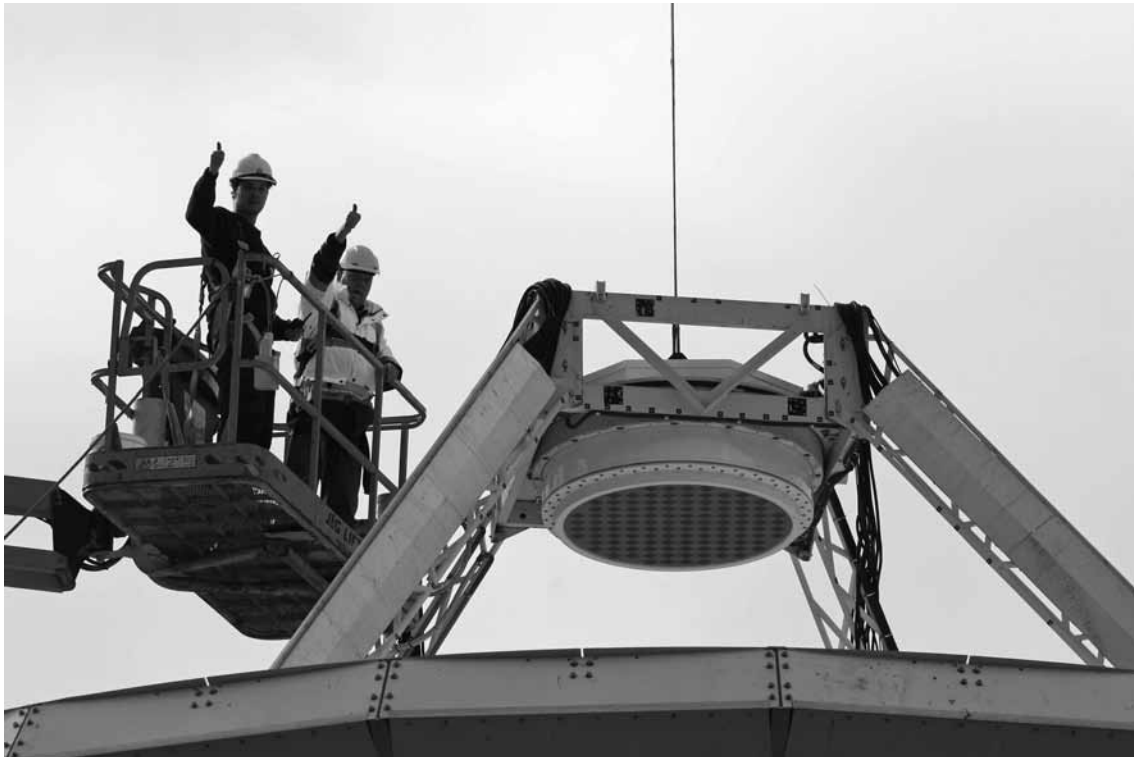
Installation of the PAF onto the Parkes Testbed Facility. Image credit: John Sarkission, CSIRO
