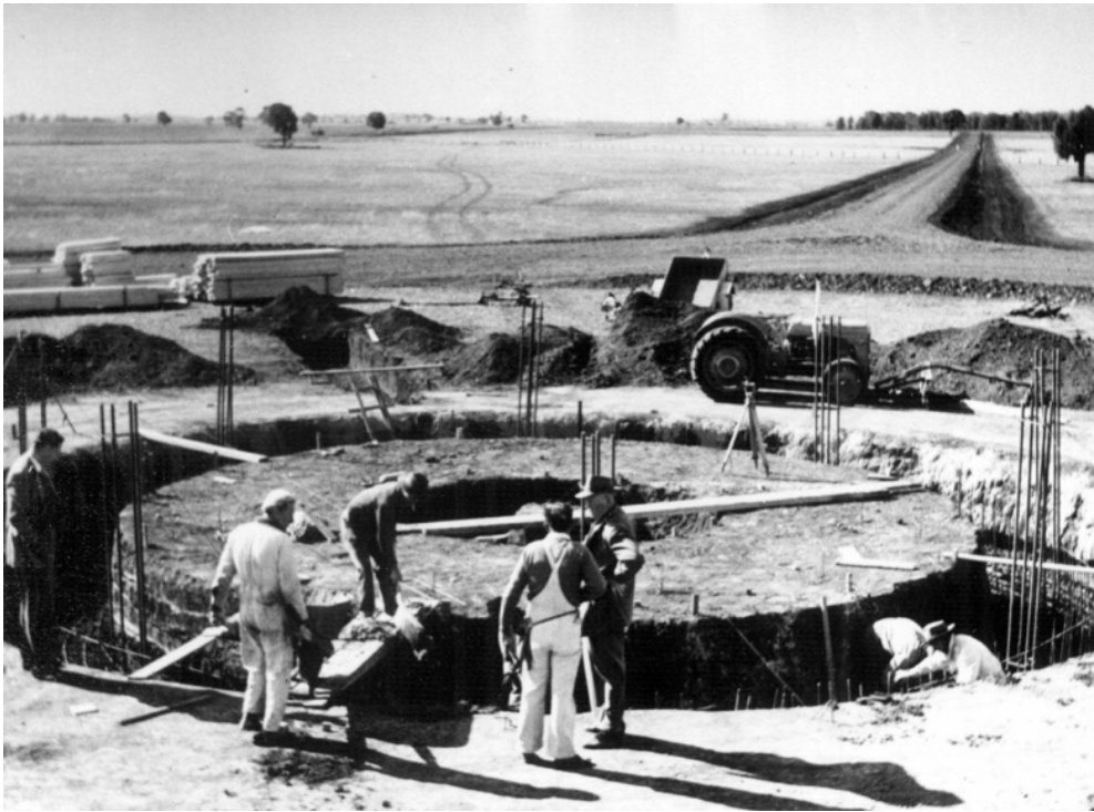
Laying the foundations for the three-storey tower. The road leads north to the site of the village area
