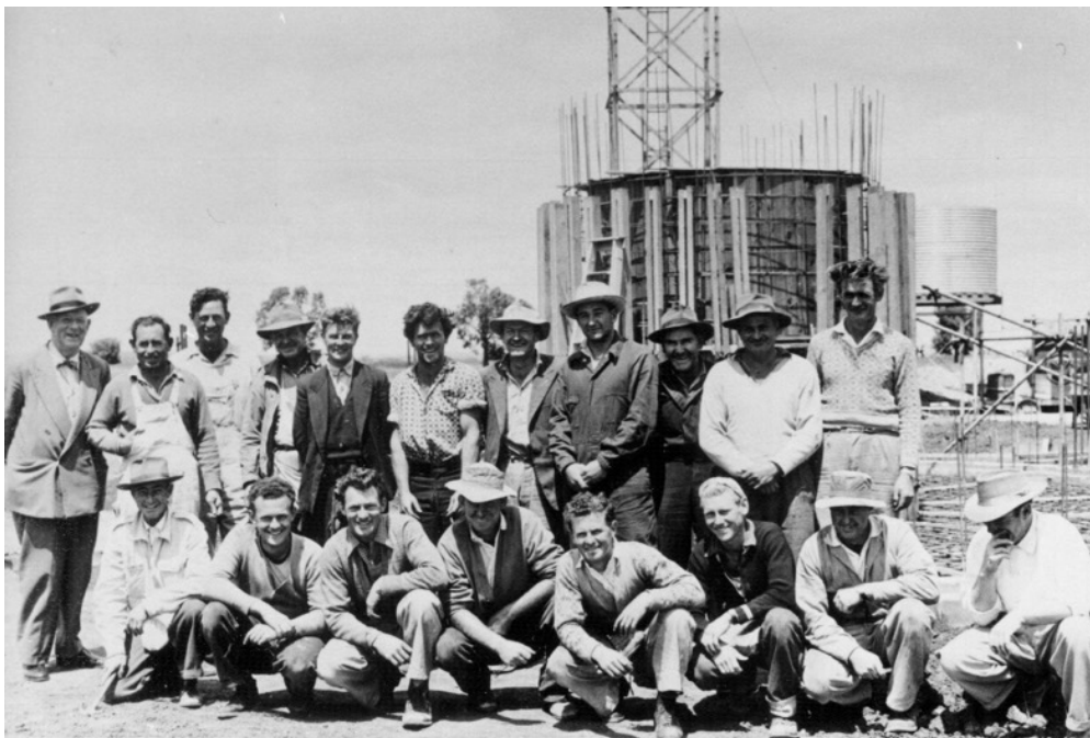
At times up to fifty construction workers were on site. MAN imported a specialist group from Germany, while most of the tradesmen were recruited from the Parkes area or brought from Sydney
